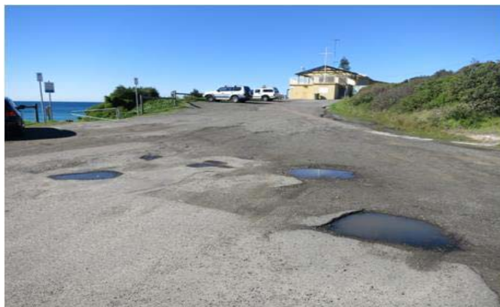
High Risk Potholes in Public Car Park
