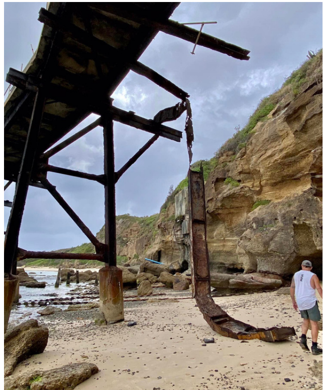
Recently a large girder fell off the jetty onto the beach
